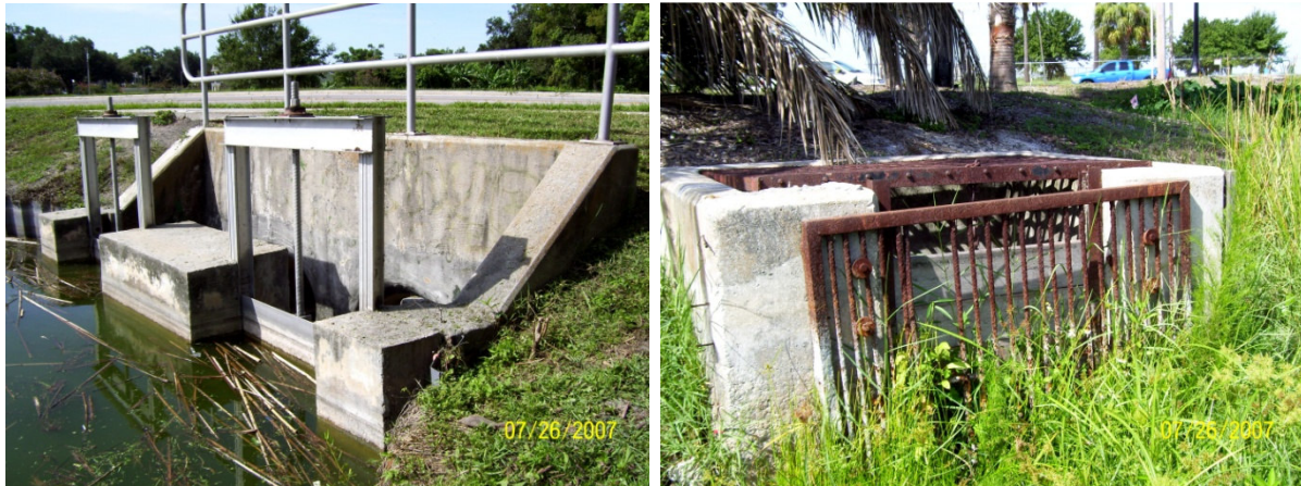
Figure 10. Adjustable water control structures. Lake Hunter, left, is a metal slide gate and Lake Wire, right, is a riser with boards. Both can be adjusted to release water through a culvert.
